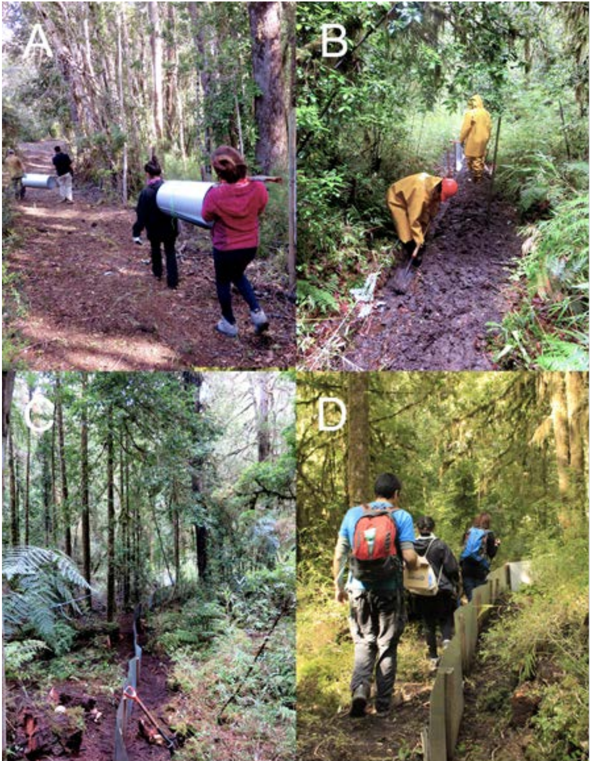
Figure 1. Installation of the exclusionary fences, a possible mitigation action against chytridiomycosis in Darwin's frog populations. In A) fieldworkers move the aluminium sheets used to build the enclosures. In B) a fieldworker is digging the ditch required for the fence during a day of harsh weather. Fences that have been successfully installed are shown in C and D.
